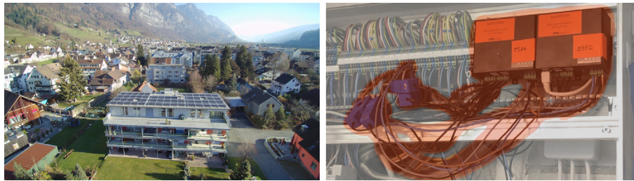
Fig. 2. Photos from the Walenstadt microgrid. The left picture shows the large prosumer apartment building with seven apartment units, a 35 kW PV system, and a 23 kWh battery. The right picture shows two SmartPi devices and attached current transformers (in red) installed in a circuit breaker box in a single family prosumer building. (For interpretation of the references to colour in this figure legend, the reader is referred to the web version of this article.)
